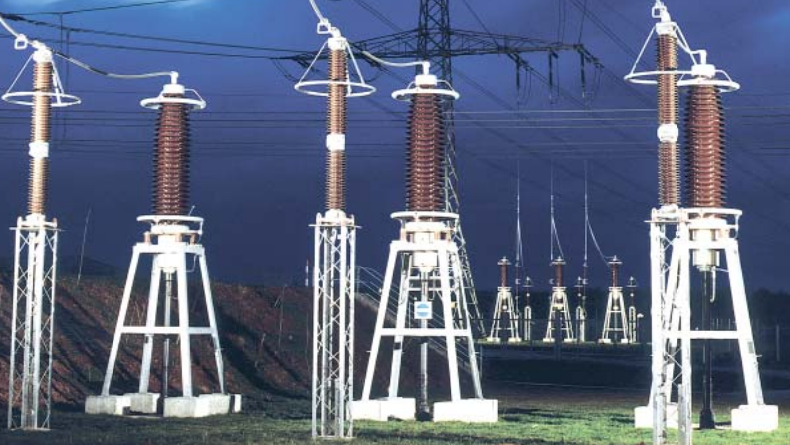
LIBERALISATION OF THE ELECTRICITY MARKET PROVIDED SUSTAINED STIMULUS TO INNOVATION AND RATIONALISATION
